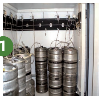
1 Glycol Beer Cold Room
