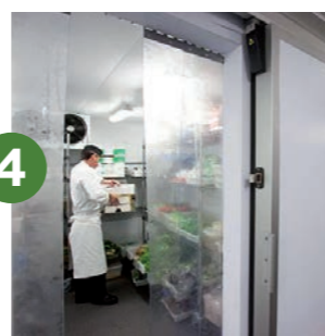
4 Glycol Food Cold Room
