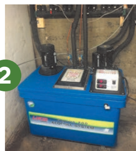
2 Glycol Tank & Manifold
